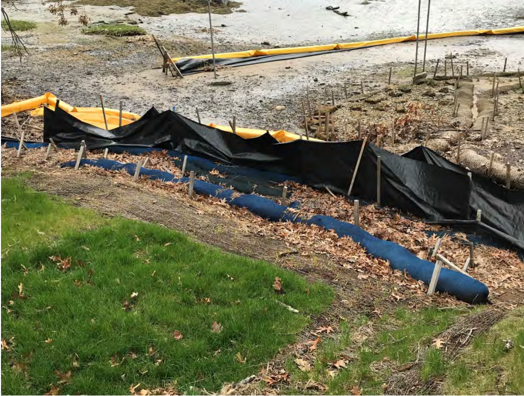
Fig 11: Toe of the slope at Gundalow Landing/east side of the bay. Viewing south. (05-04-21)
