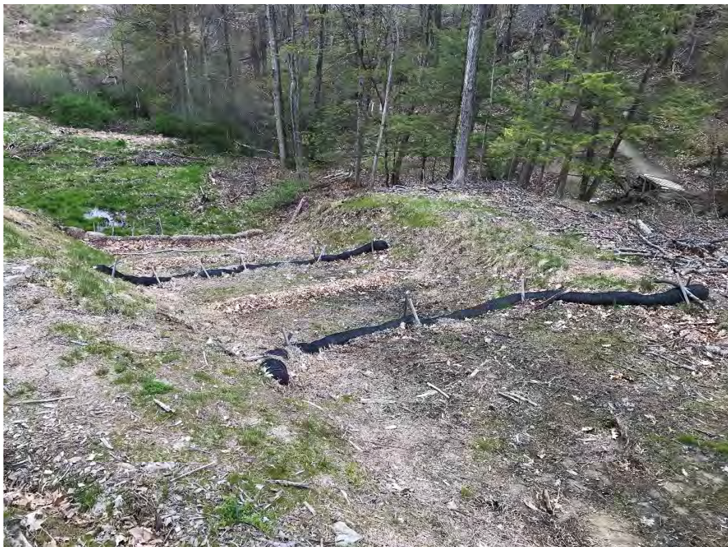
Fig 8: Lower portion of slope between Strs. 28 and 29. Viewing northeast. (05-04-21)
