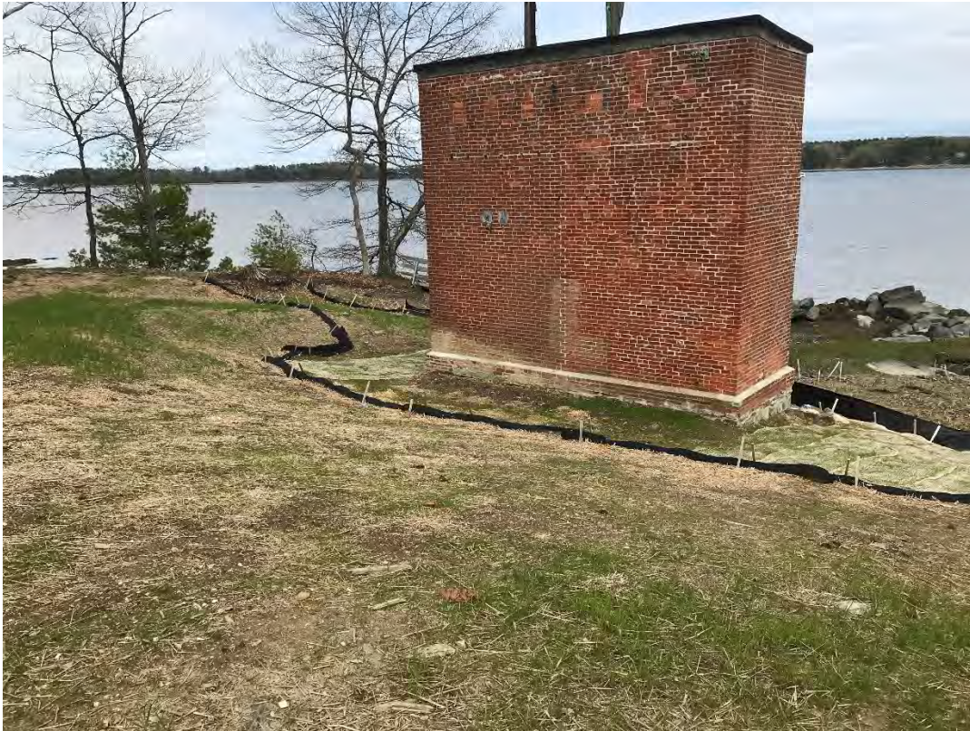
Fig 1: Slope leading down to cable house and salt marsh restoration at the west side of the bay. Viewing northeast. (05-04-21)
