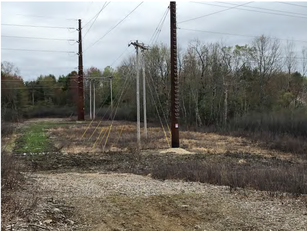
Fig 14: Str. 47 work area with adjacent access route, wetland DW56, and Str. 48 work area in background. Viewing south. (05-04-21)
